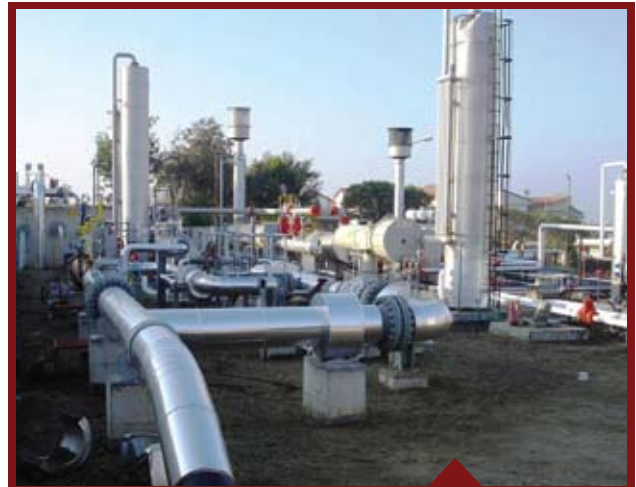
Kuzey Marmara Natural Gas Process Facilities
